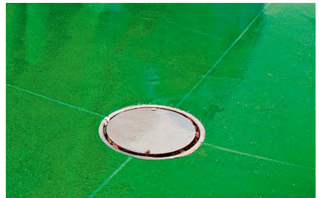
Figure 1. Gulley with screed to falls. Such joints are unnecessary.
