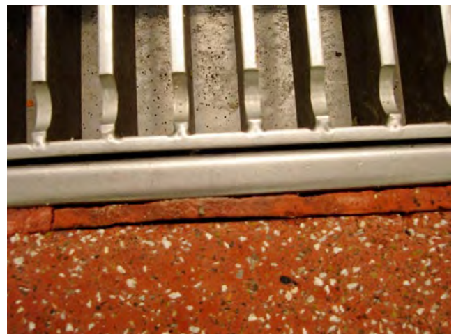
Figure 2. Hygienic failure example.
