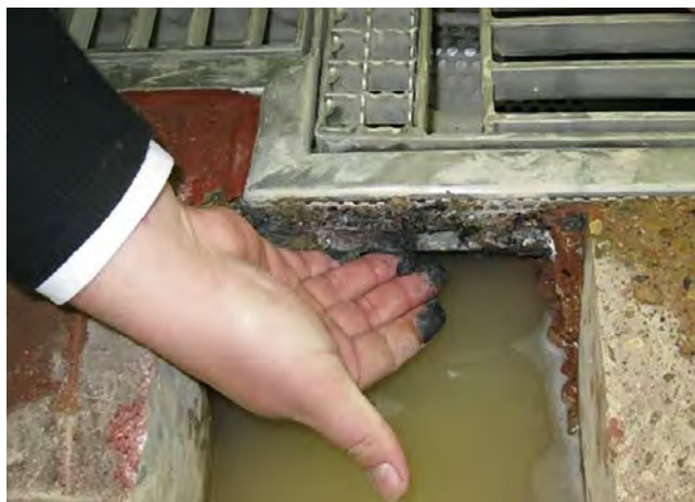
Figure 4. Pathogen build-up after long-term structural failure.
