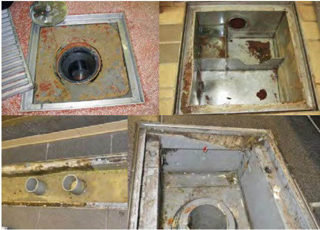
Figure 3. Poor drainage component design includes metal-to-metal contact, gaps, sharp corners, and non-drainable areas.
