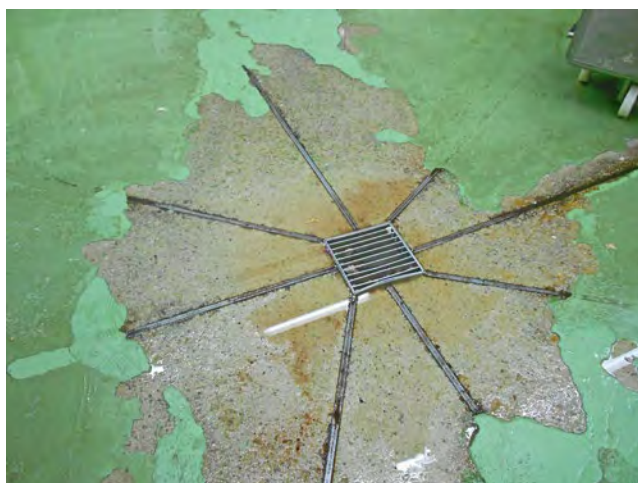
Figure 3. Built to fail; no one designed the floor like this, it just got built that way due to lack of site control.
