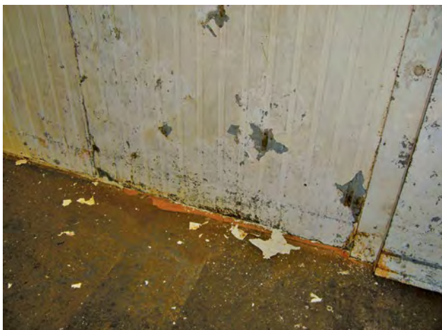
Figure 1. Damaged and corroded steel sandwich panels.
