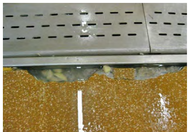
Figure 3. Example of structural floor failure.
