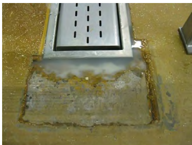
Figure 5. Failure of a poor-quality repair.
