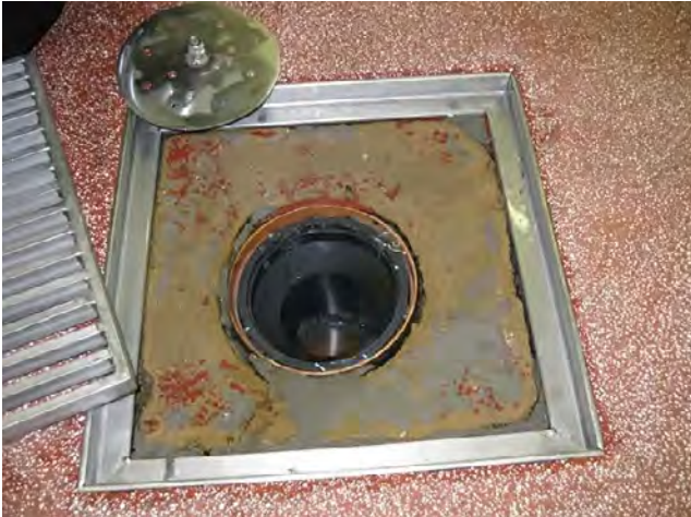
Figure 7. Example of a poorly fabricated drainage gully.
