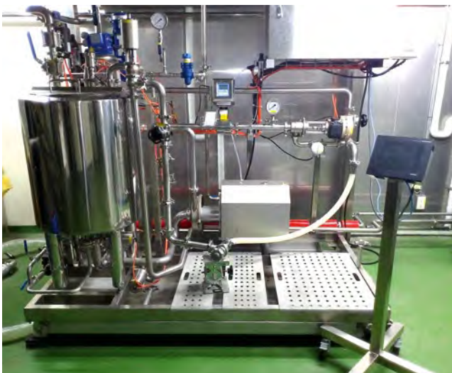
The CIP test rig at the experiment plant for hygienic engineering.
